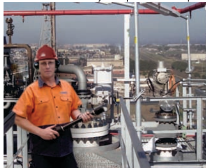
BAZOOKA & Shroud used in Industrial Maintenance Coated Style for prevention of sparks
